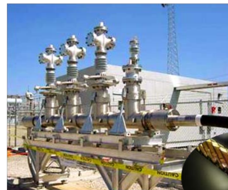
Triaxial superconducting cable installed at AEP Bixby
